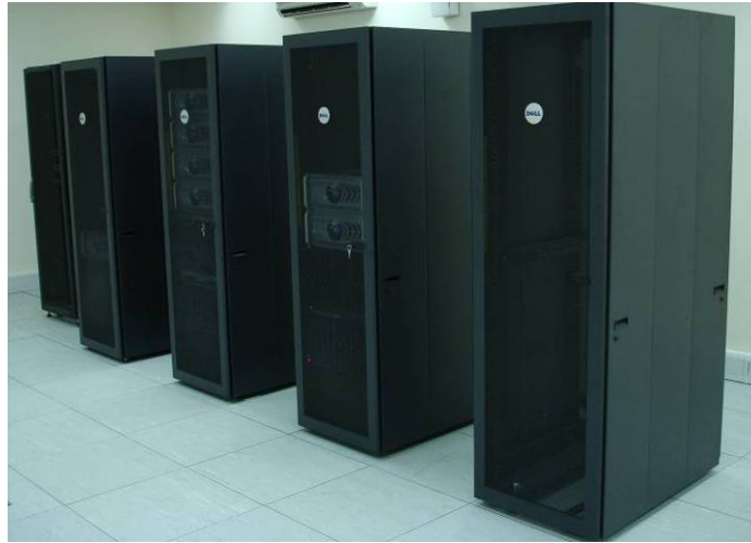
Figure 9: The Data Centre of distributed deployment - empty rack space due to installation in progress
