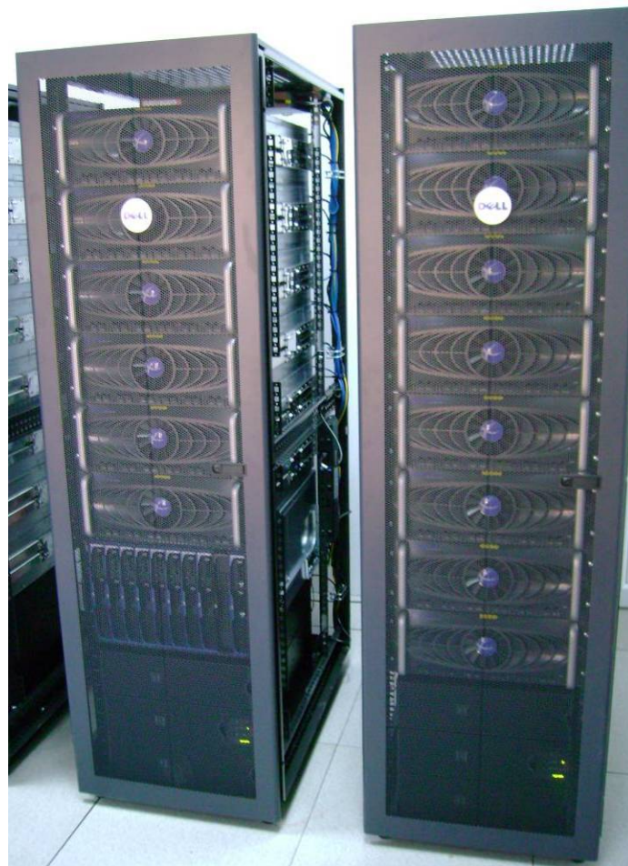
Figure 10: Fully populated processing and storage racks
