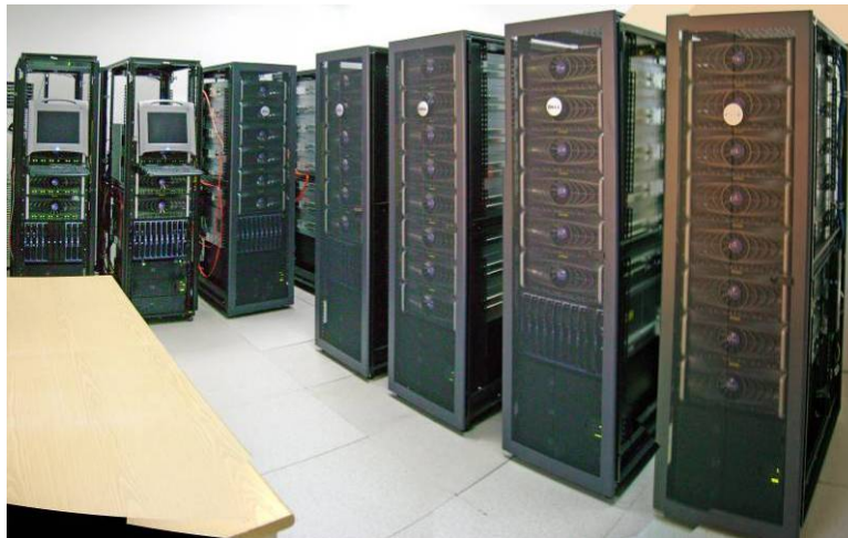
Figure 8: Zebra system during installation – note storage units in 5 racks to the right
